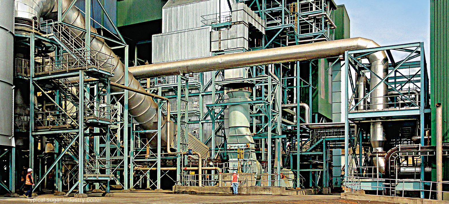
typical sugar industry boiler
